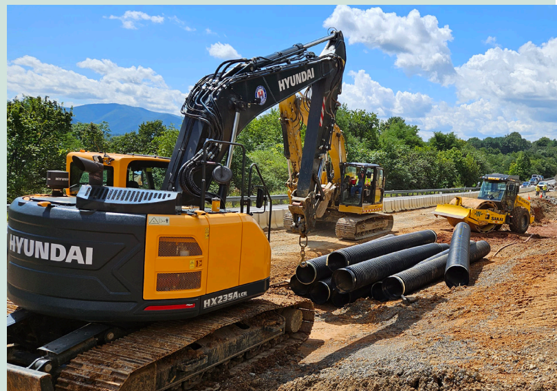
Bridge replacement and widening work are taking place near exit 137 at Salem.
