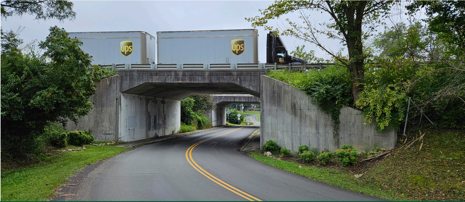
Adding a third travel lane requires widening the I-81 southbound bridge over Old Dominion Road.
