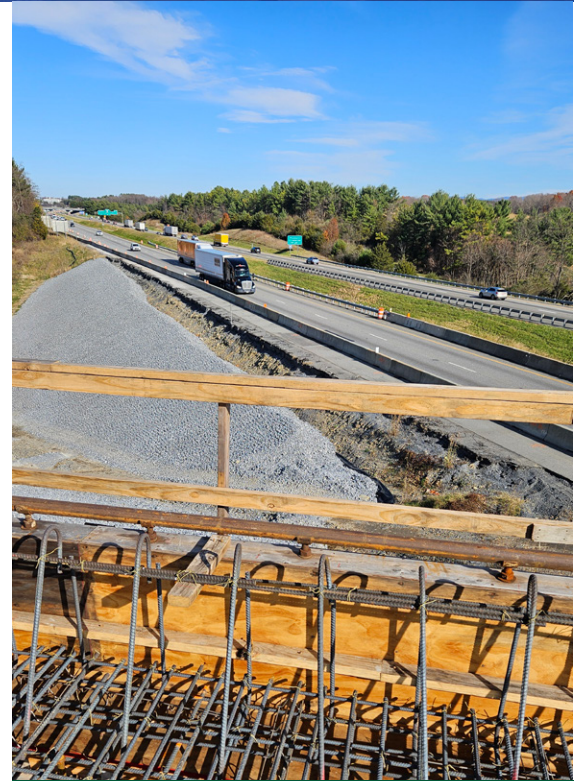
The new Route 635 bridge over I-81 will allow construction of an auxiliary lane
